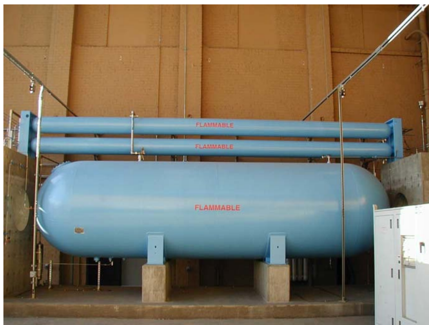
Figure 2.3. Hydrogen low-pressure storage vessel is the large tank on the bottom and the two high-pressure storage vessels are on top.
