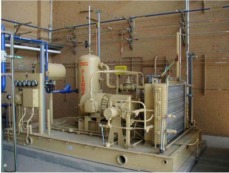
Figure 3.2. Gemini - main CNG compressor.
