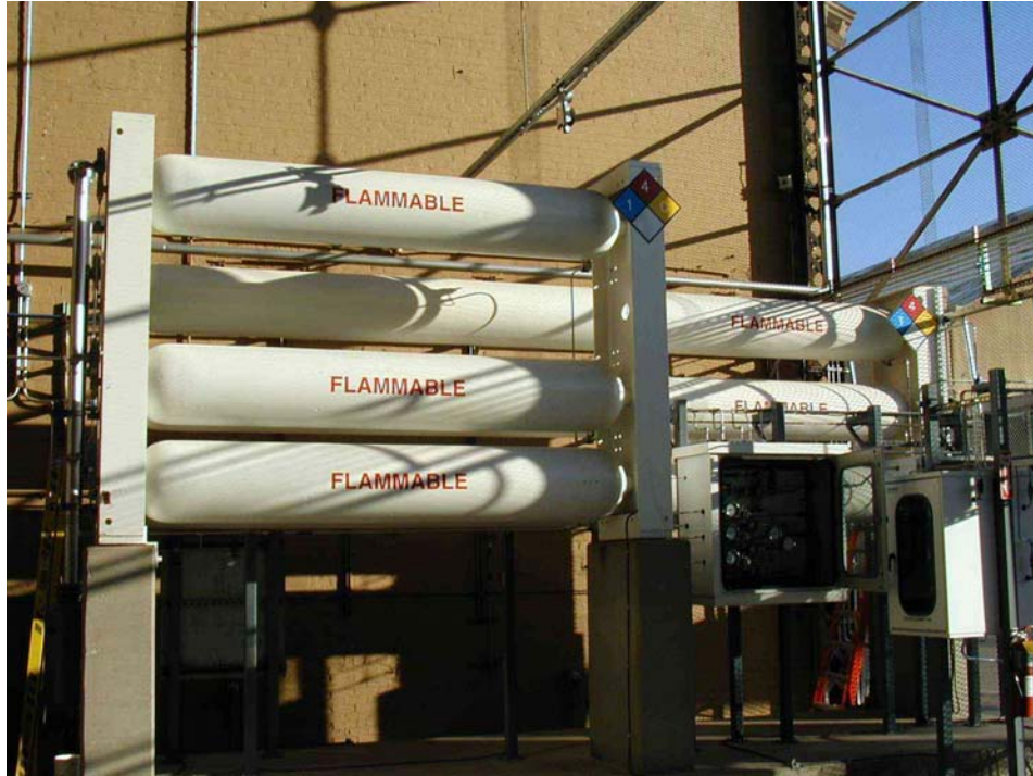
Figure 3.3. CNG storage tanks. The top tank is the high-pressure tank and the two lower tanks are the medium-pressure tanks in the near rack. The three low-pressure tanks are in the far rack.
